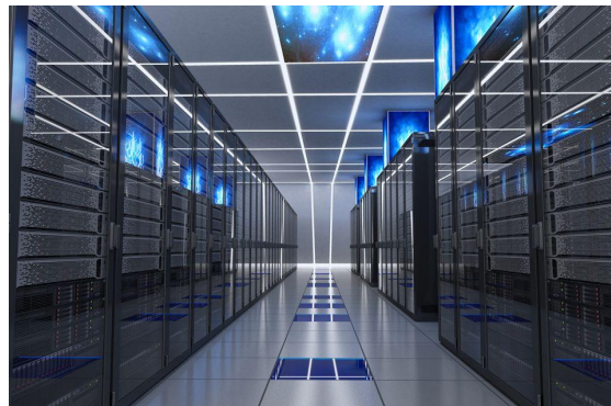
HPC Servers/Data Centers
